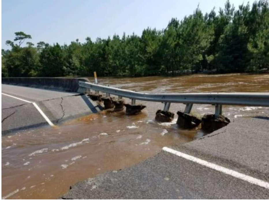
Fig. 10 On September 1, 2017, high flow resulting from precipitation during Hurricane Harvey washed out part of the US96 Village Creek bridge (survey site 6 on the map). The high-flow event and associated scour decimated what was formerly the largest documented bed of Fusconaia sp. in the region.
